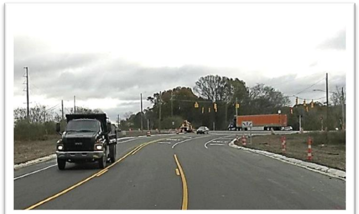
The final layer of asphalt is one of the last steps in finishing the project
